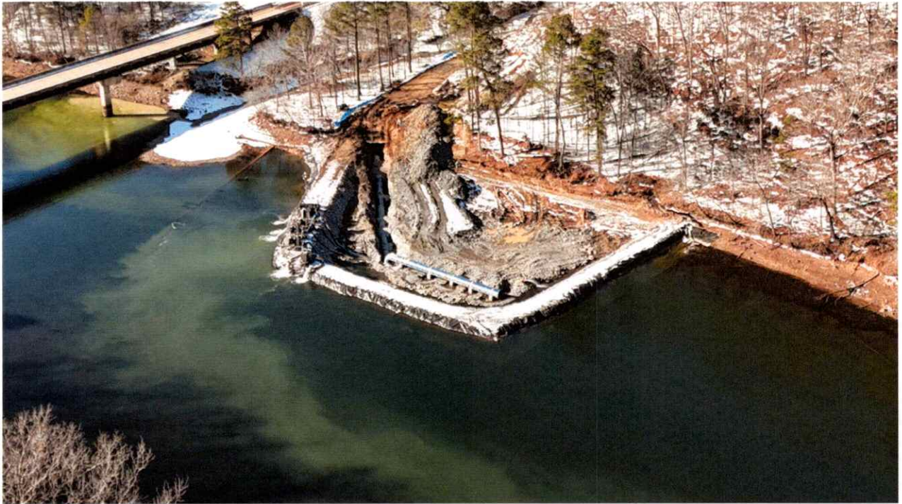
Davidson Drive WWTP Discharge
